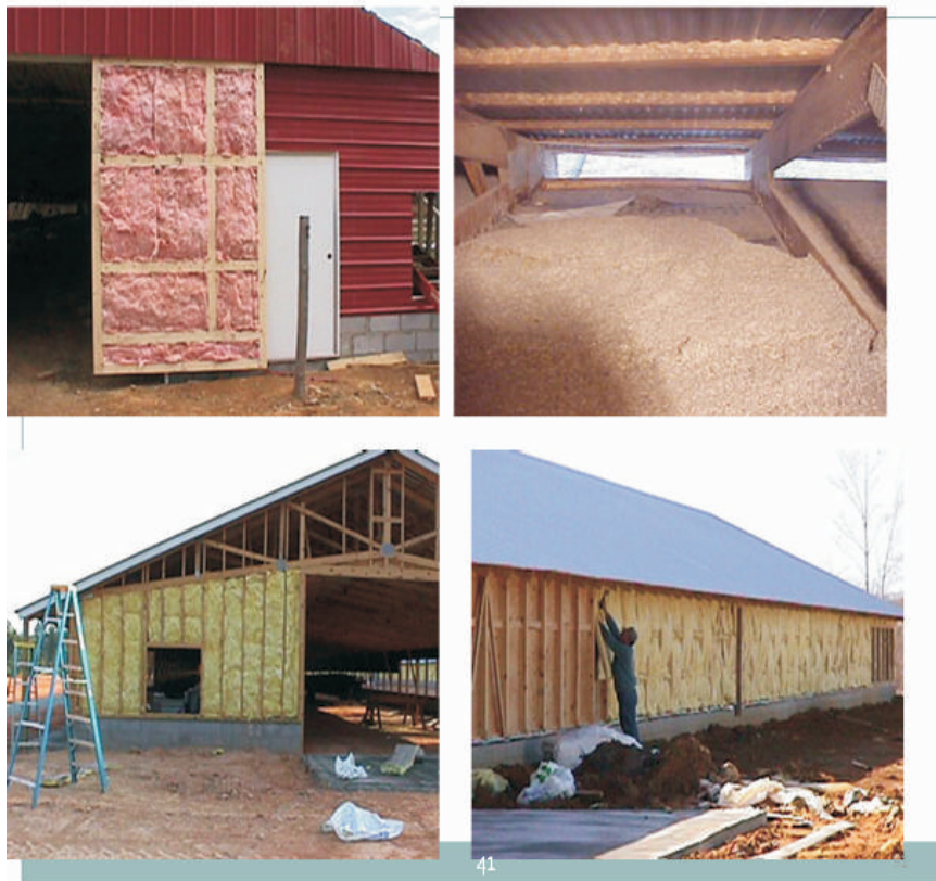
Figure 13: Different insulation materials used for poultry houses
